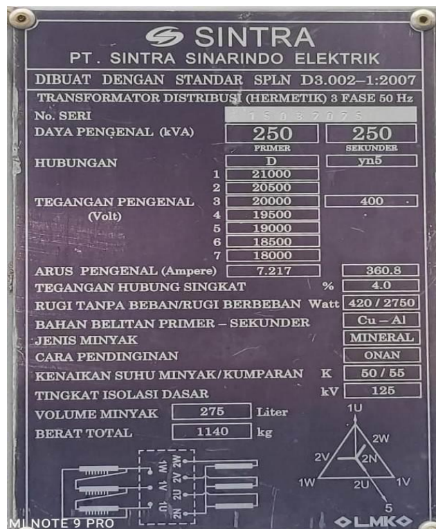
Gambar 4.2 Nameplate Transformator 250kVA No.Seri15037075
